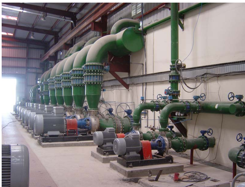
Figure 3.10 Complete Pumping Station built by Turbosan
